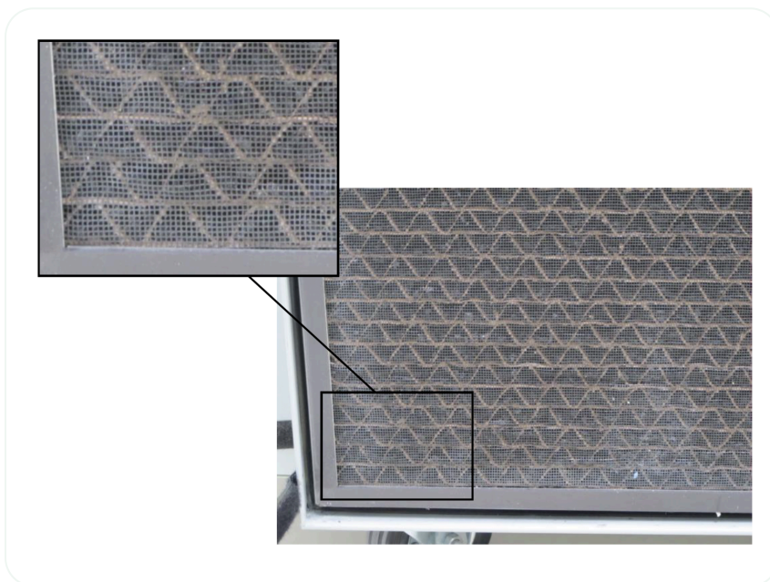
Fig. 4.1.2.1 Beginning patina formation. This filter does not yet need to be replaced.
